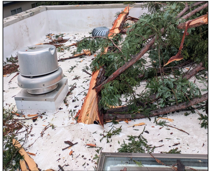
One of three, a redwood tree splinter penetrates the roof of the Msgr. Fahey Parish Center. Photo by Kurt Amman
