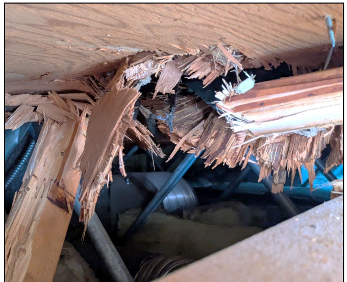
Roof truss/joist, above the women's bathroom, sheared by Redwood tree spear. Photo by Kurt Amman
